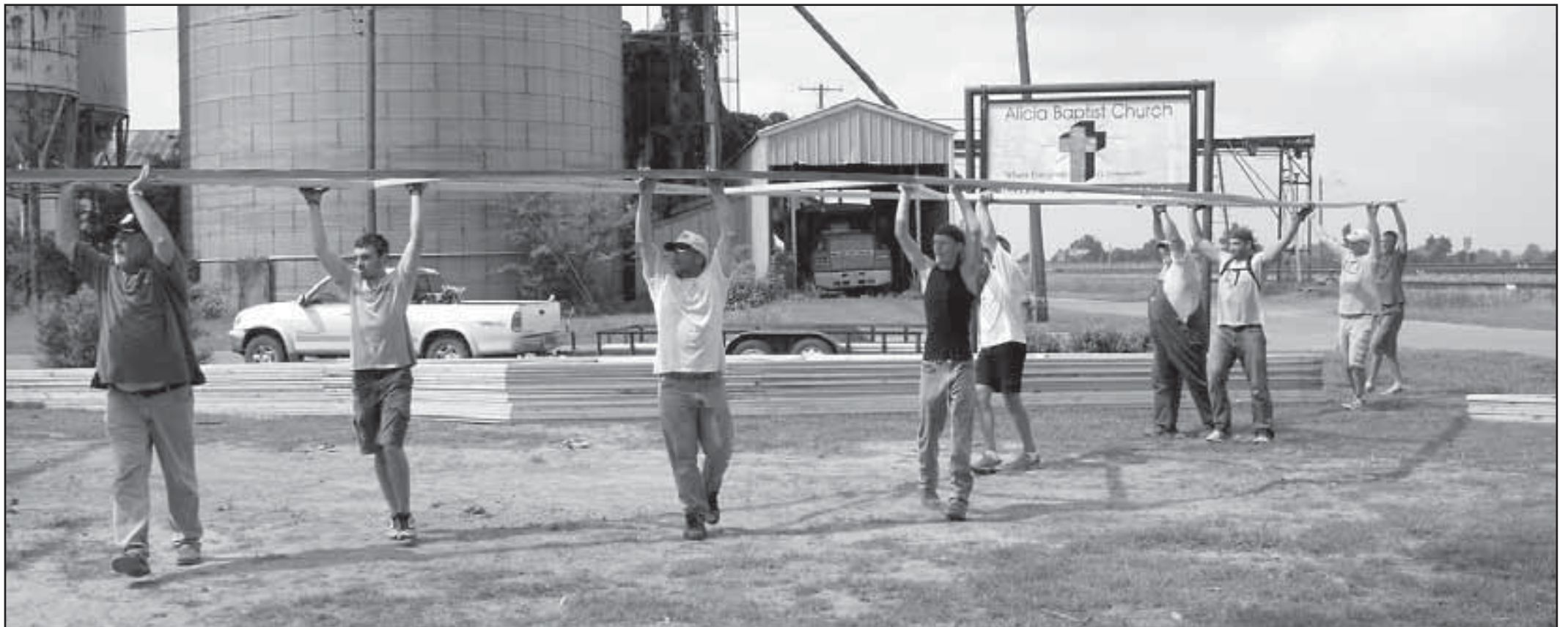
A group of men carry a truss for the roof of the new building. Volunteer labor and donated materials have made the project possible.
