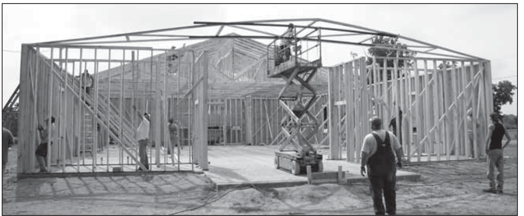
Volunteers work to frame up the new building at Alicia Baptist Church. The building will house a sanctuary, freeing up space in the current church building to be used for outreach ministries.
